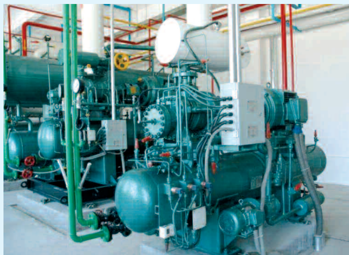
Figure 2. \text{CO}_2 compressor unit
