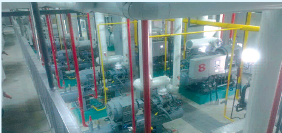
Figure 8. Corner of \text{CO}_2 engine room
