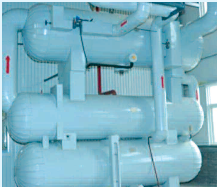
Figure 3. CO 2 Auxiliary unit
