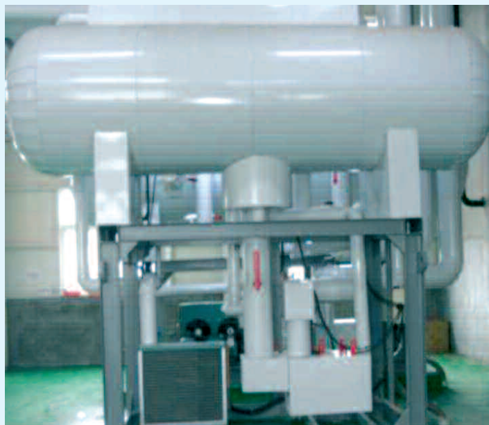
Figure 4. CO 2 barrel pump unit
